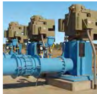
Raw water pumps
