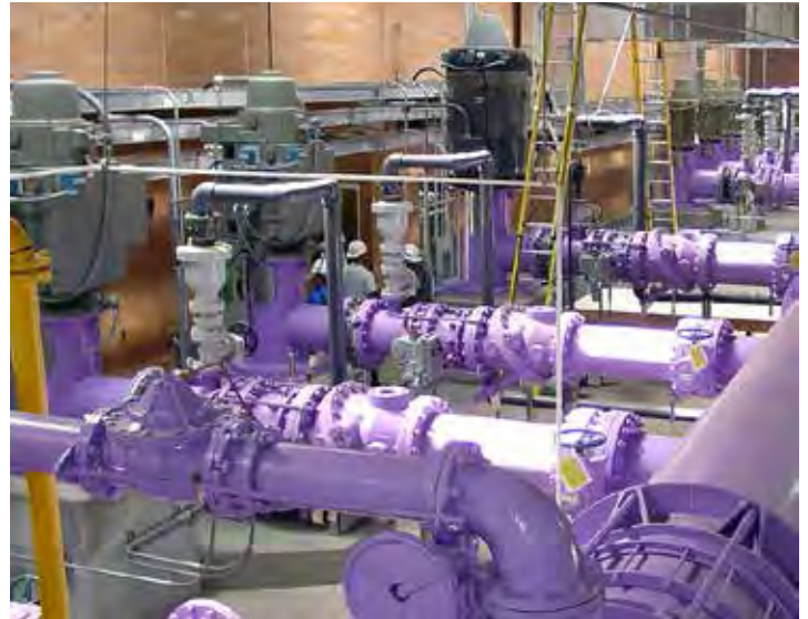
Finished water pumps
