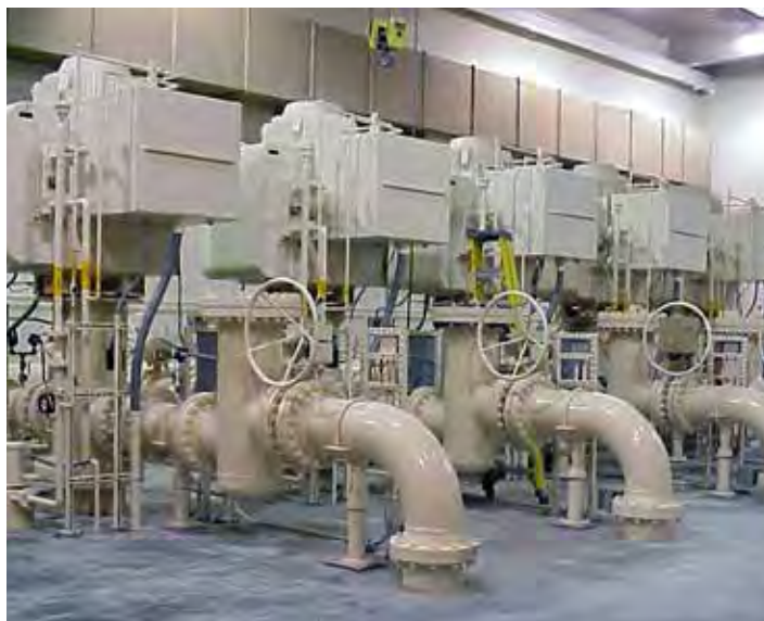
Recycled water pumps
